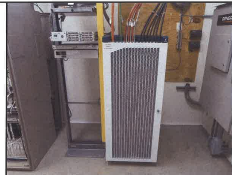
B EXISTING LTE EQUIPMENT CABINET
