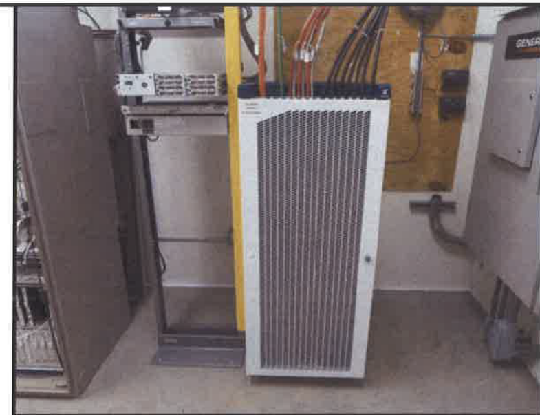
B EXISTING LTE EQUIPMENT CABINET
