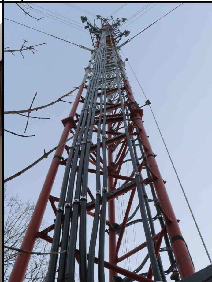
F CABLE ROUTING UP TOWER FACE
