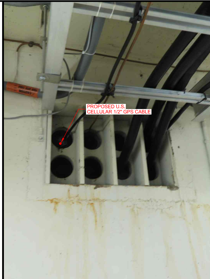
C SHELTER COAX PORT (SHELTER INTERIOR)
