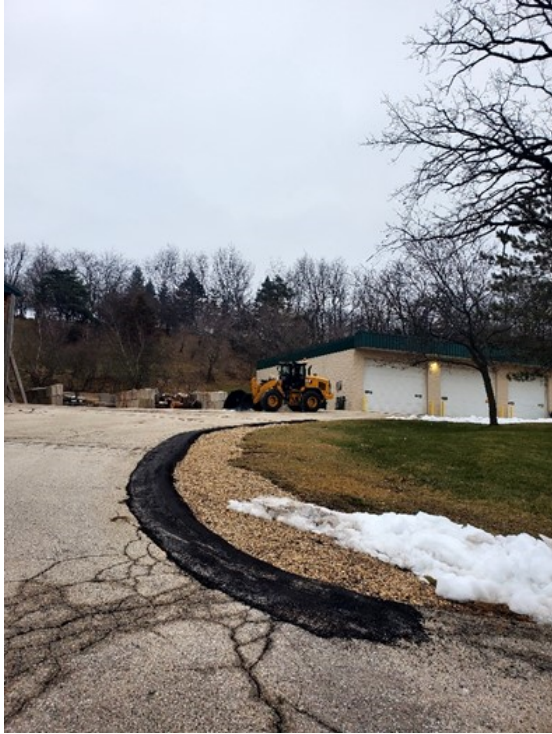
Erosion Area of Concern Resolved
