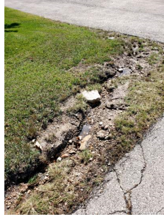
Erosion Area of Concern
