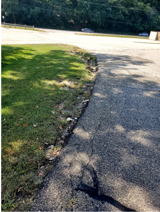
Erosion Area of Concern
