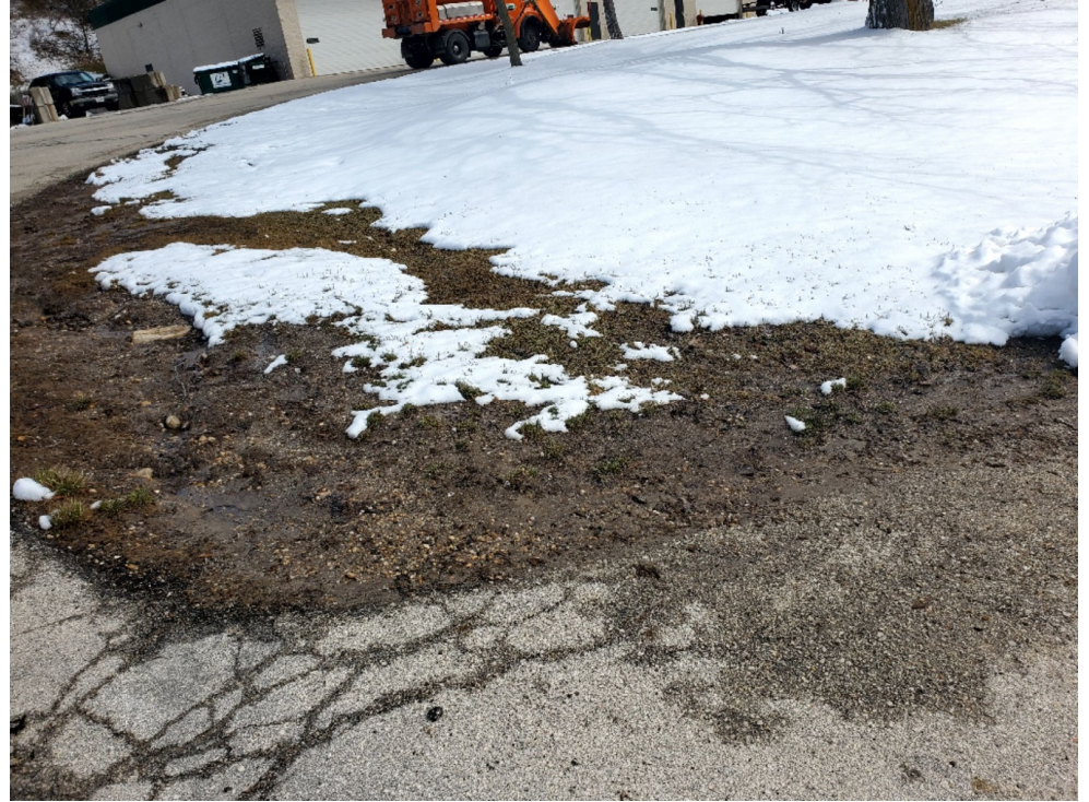
Erosion Area of Concern
